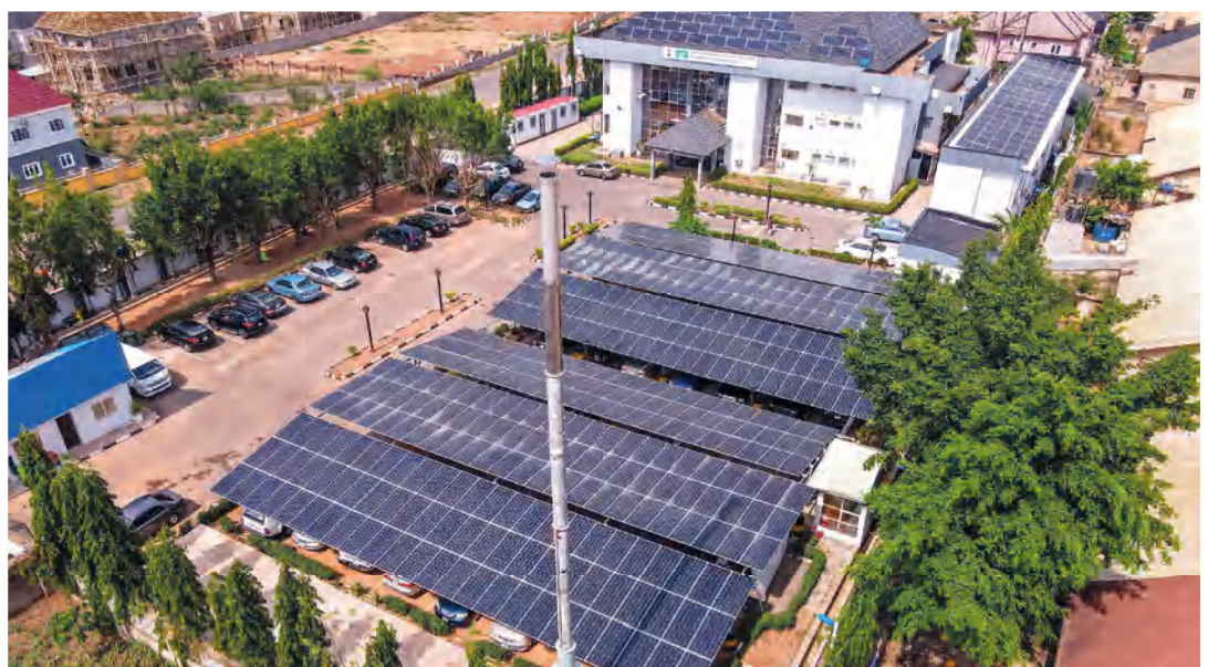
Solar panel systems installed at NRL, Gaduwa
