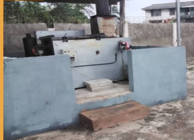
Incinerator house with incinerator for burning waste
