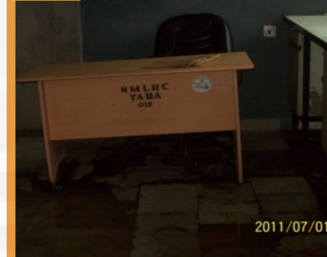
Damaged floor as a result of constant water seepage into wash-up room
