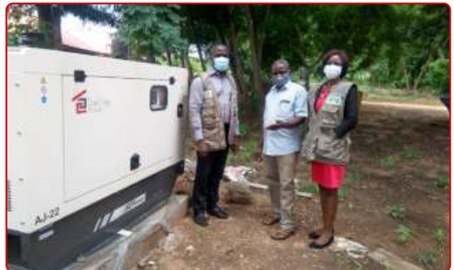
ONE OF 37 20KVA POWER GENERATING SETS PROCURED BY THE REDISSE PROJECT TO SUPPORT OPERATIONS AT THE STATE PHECCS ACROSS THE COUNTRY, AS PART OF COVID-19 SUPPORT AT THE SUB-NATIONAL LEVEL.
